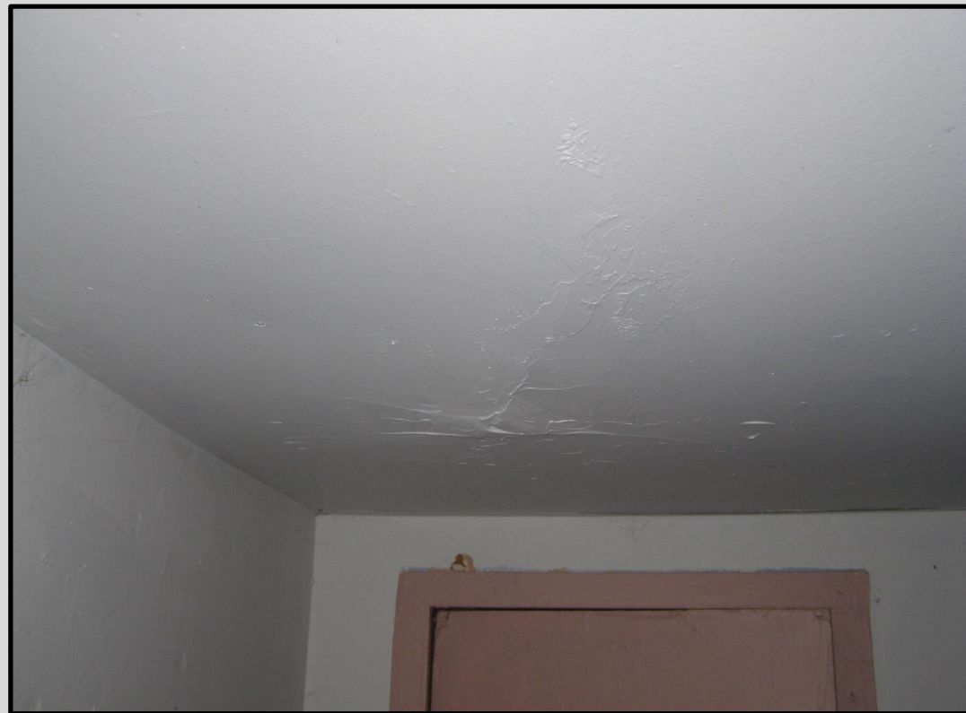
Cracked ceiling plaster. Possible roof leak
