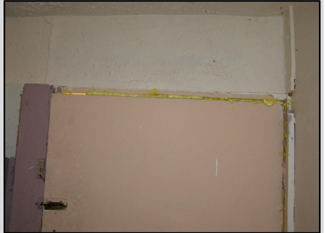
Defective exterior door. Same door as picture 10
