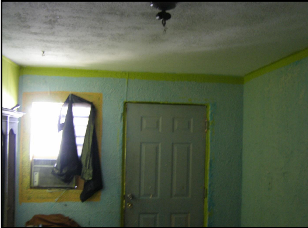
Substandard light fixture Door not weather tight
