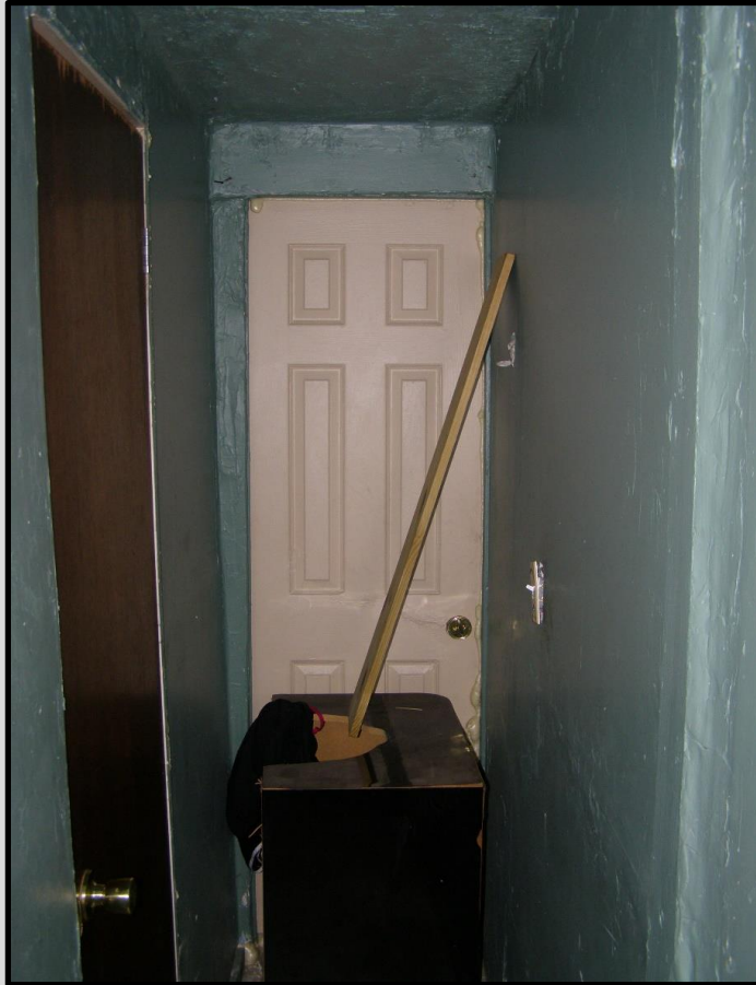
Closed off hallway to create illegal duplex
