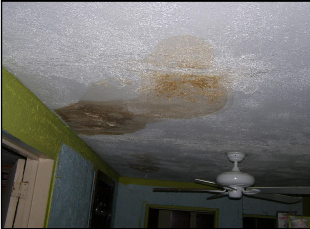
Roof defect causing water damage on ceiling
