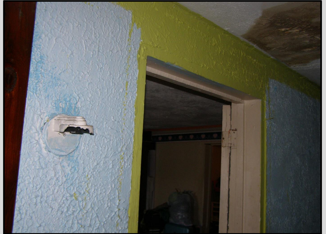
Broken light fixture
