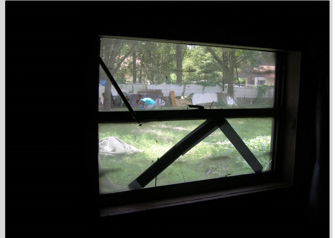
Broken bedroom window
