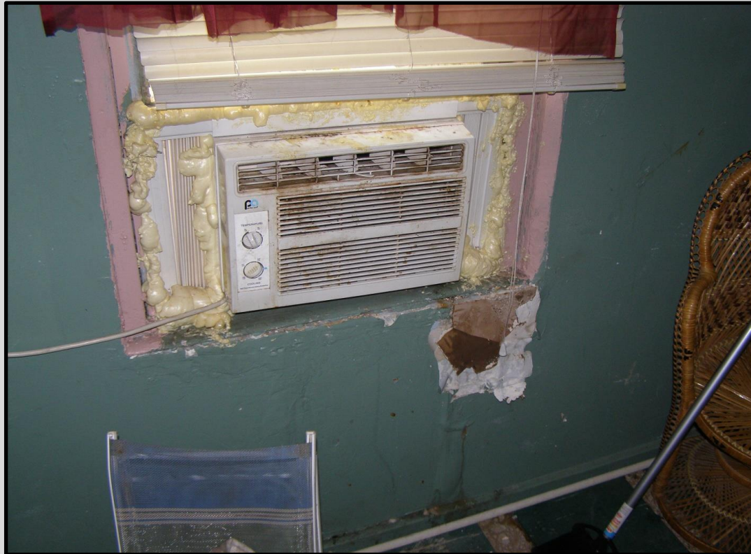
Substandard wall conditions
