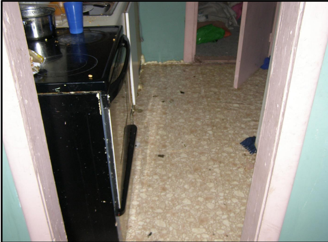
Defective interior surfaces
