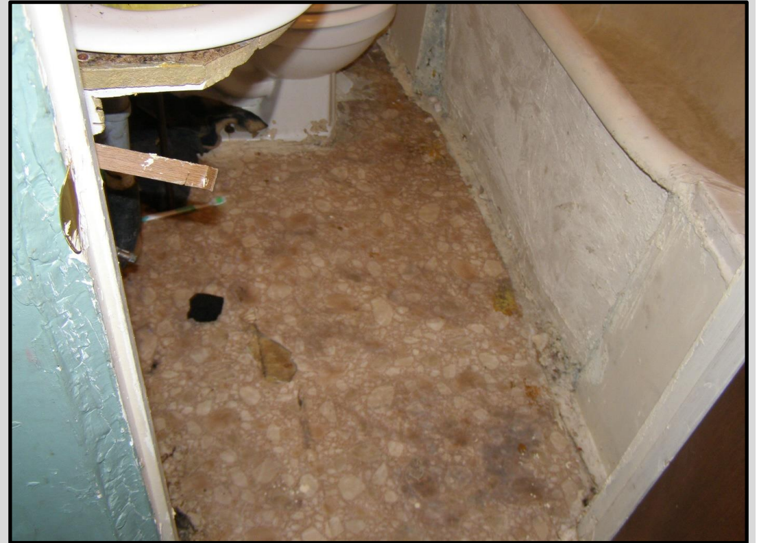
Substandard flooring conditions
