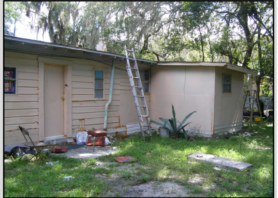
Poor exterior siding conditions
