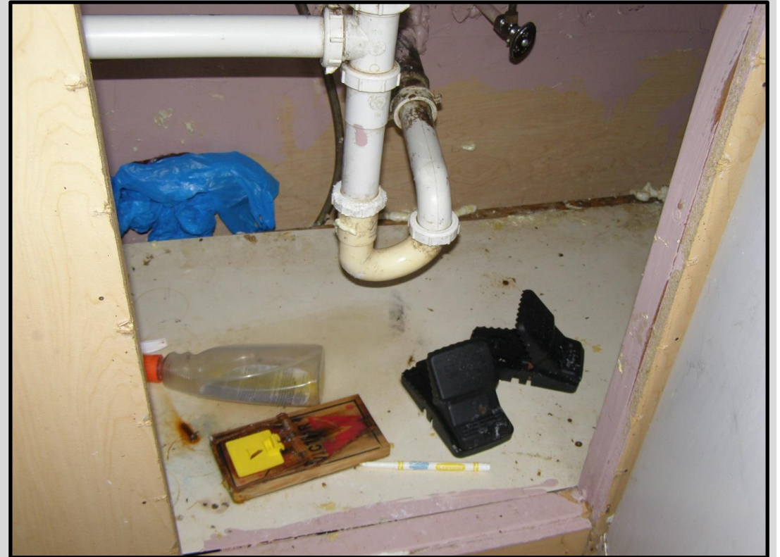
Unsanitary conditions under kitchen sign/hole in wall
