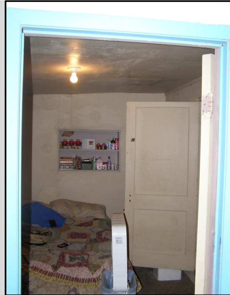
Substandard sized bedroom. No door hardware
