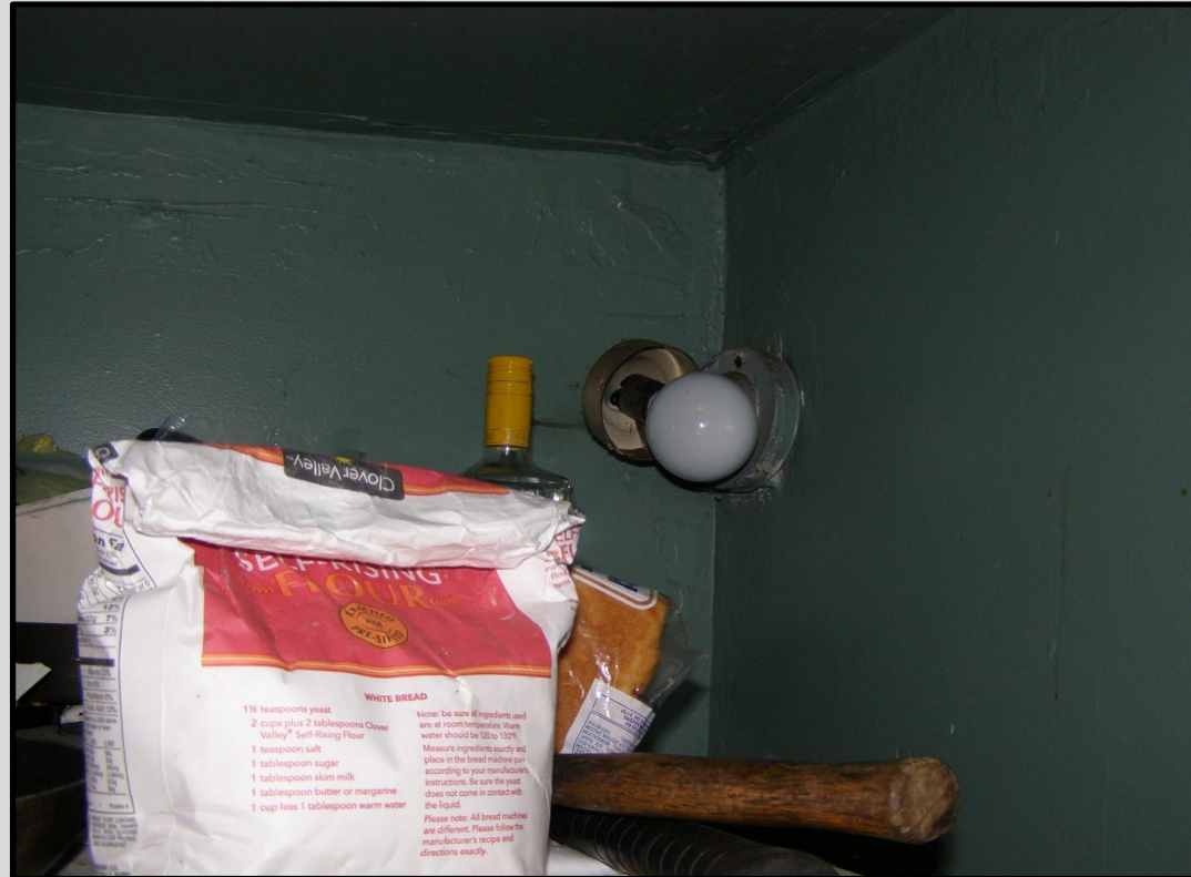
Substandard light fixture
