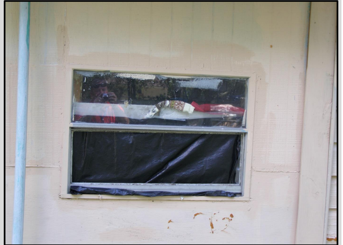
Closer view of broken kitchen window
