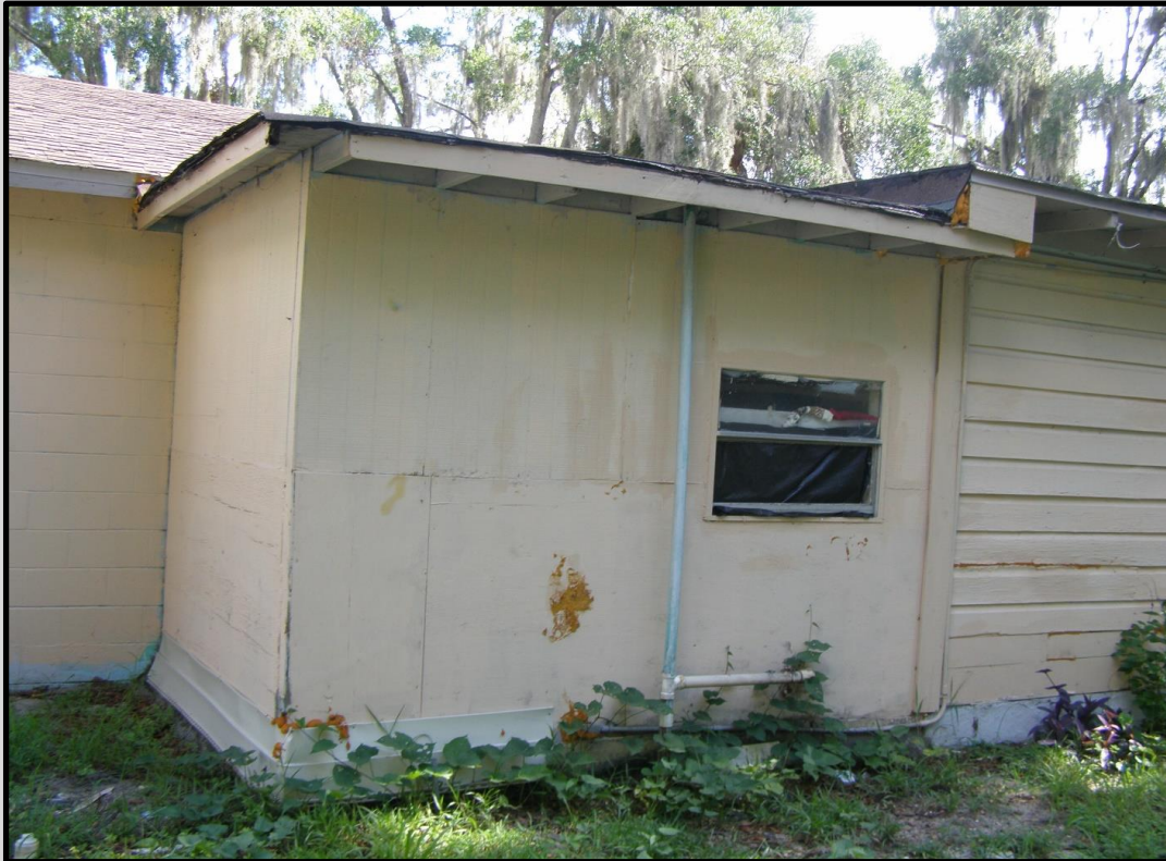
Wooden kitchen addition/broken window
