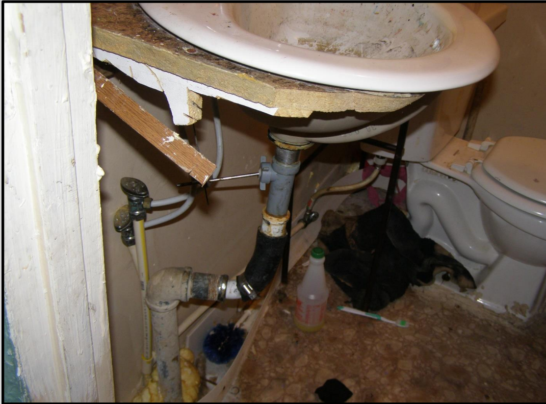
Defective plumbing fixtures, etc.
