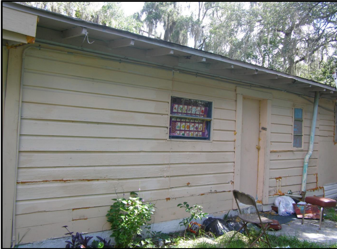
Poor exterior siding conditions
