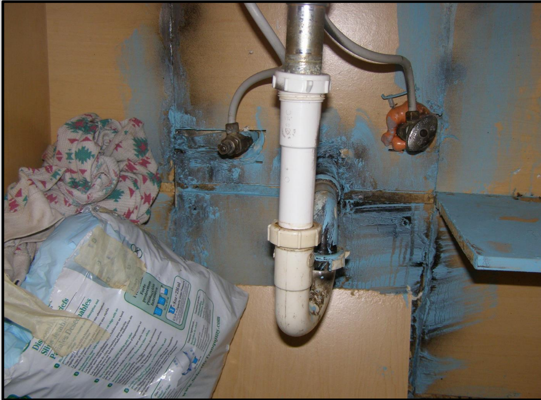
Broken plumbing valve
