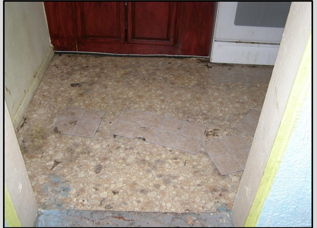
Poor flooring conditions
