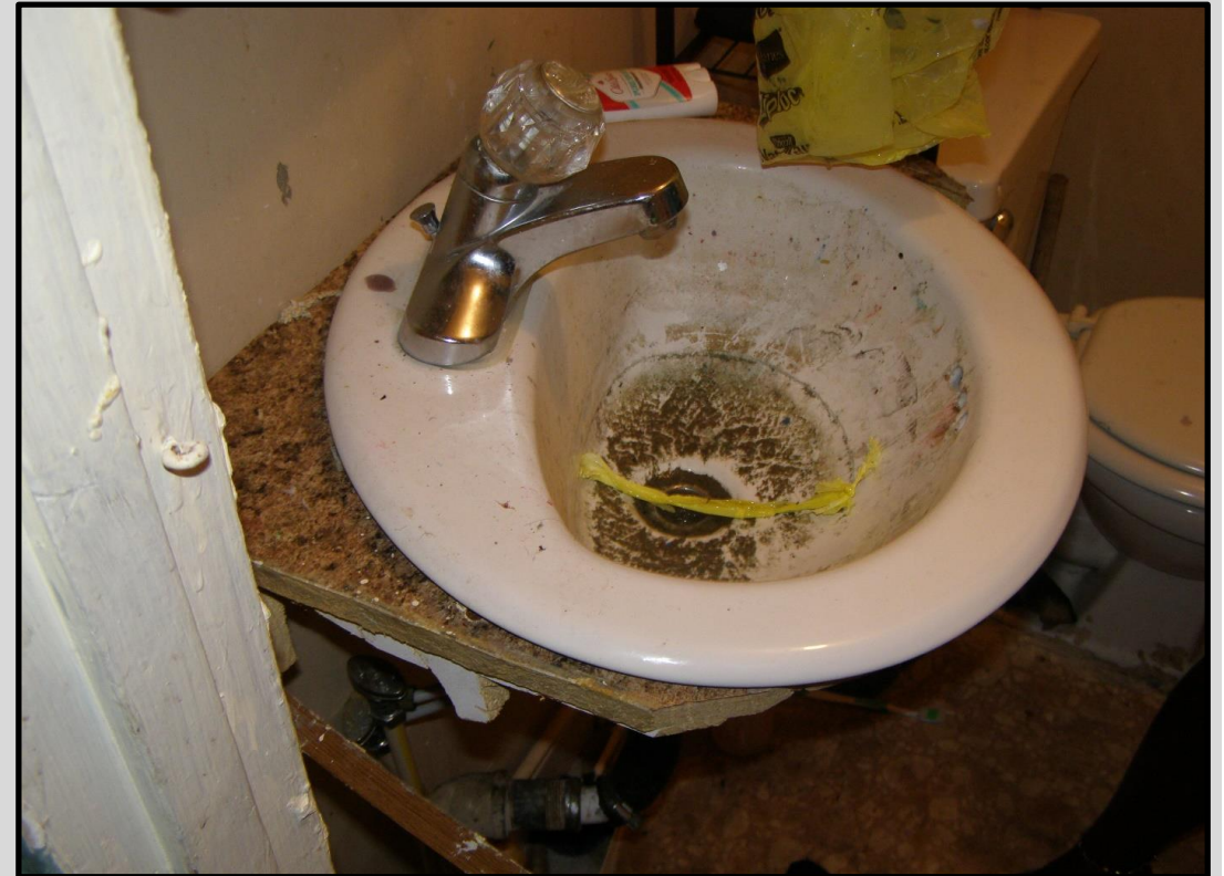
Defective plumbing fixtures, etc.
