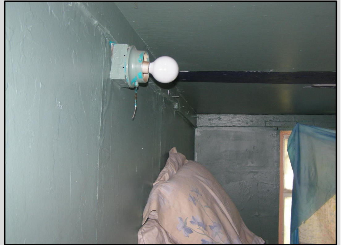
Substandard light fixture
