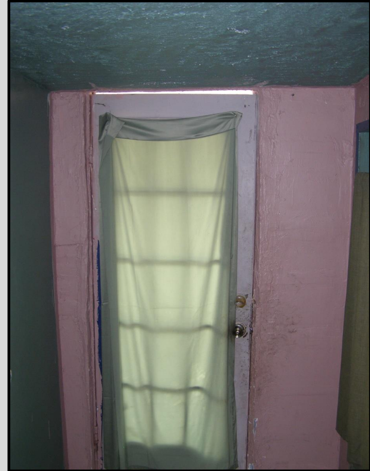
Exterior door not weather tight
