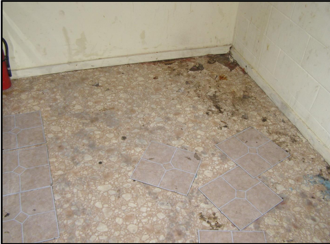
Poor/defective flooring conditions
