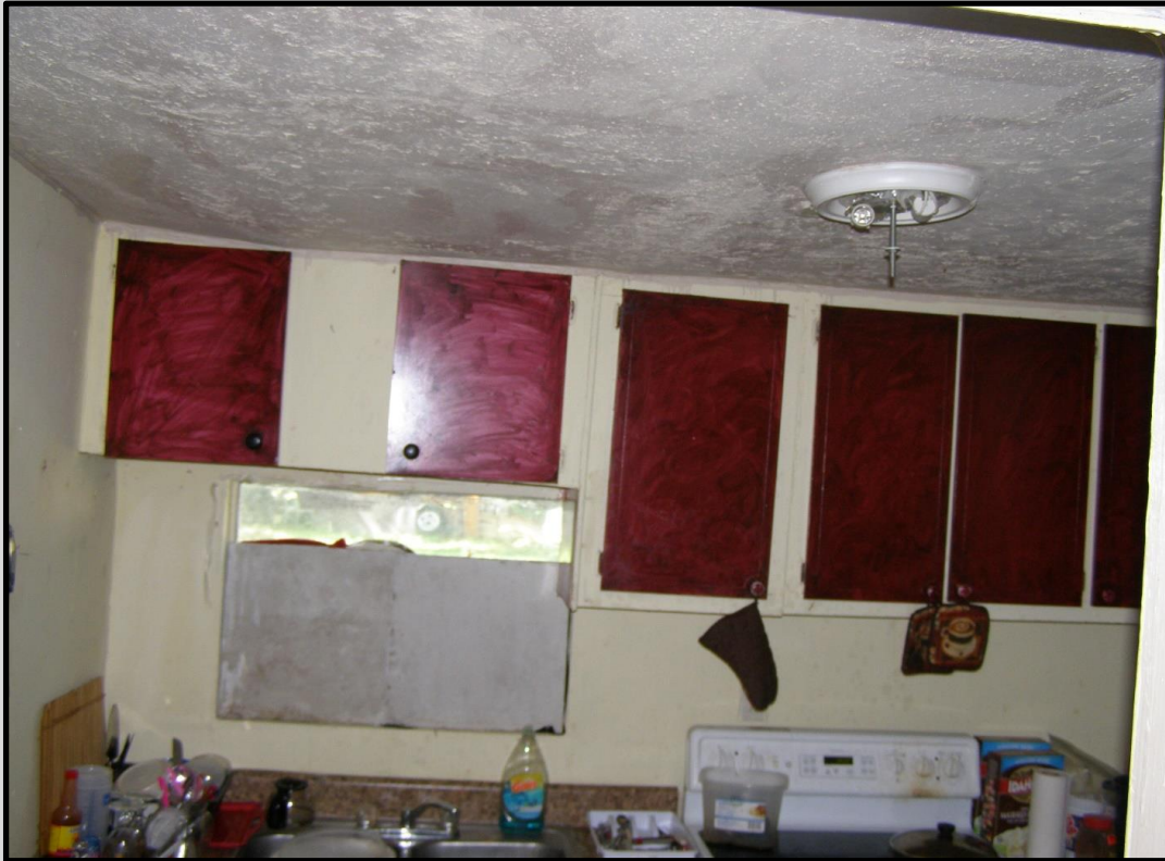
Substandard light fixture Boarded Window No electrical power in kitchen
