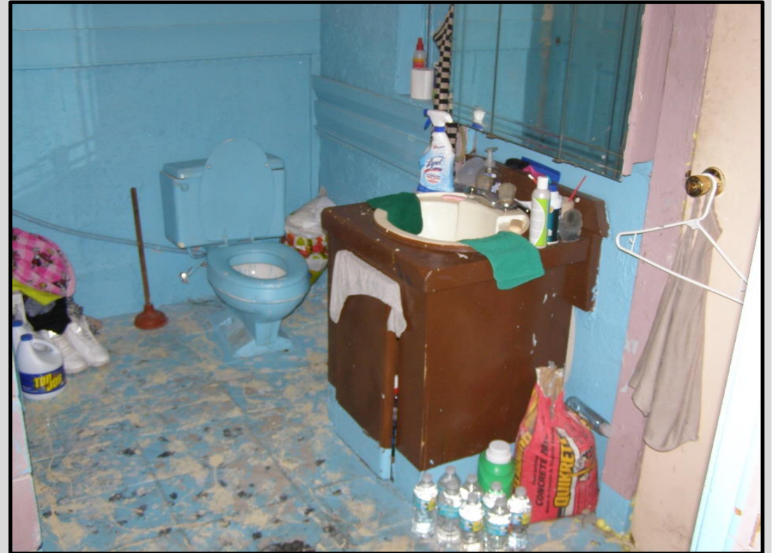
Poor floor conditions, Defective exterior door No cold water to sink and another bathroom (no picture) had no hot water
