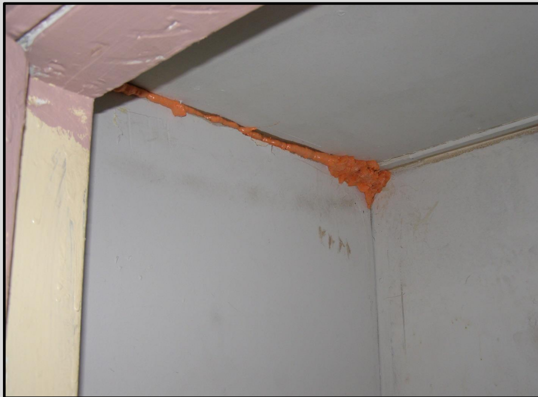
Defective wall/ceiling conditions
