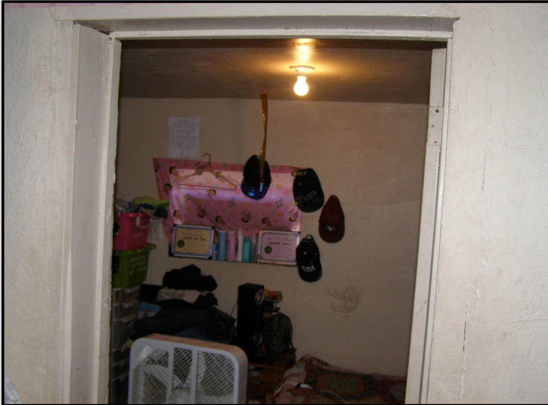
Improperly sized bedroom egress window
